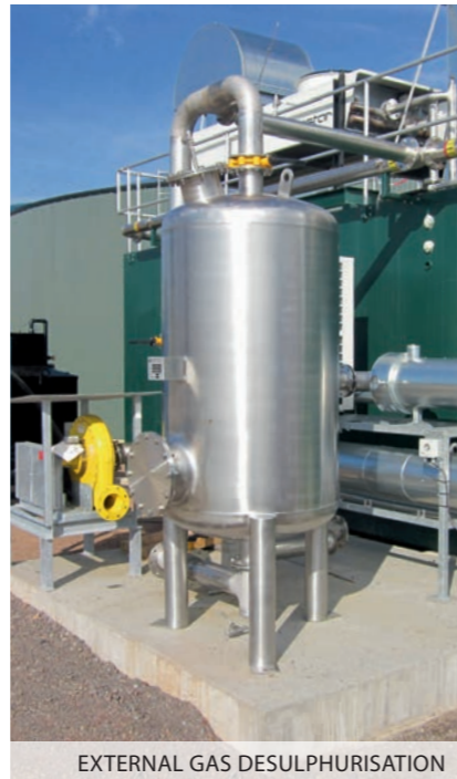
EXTERNAL GAS DESULPHURISATION
