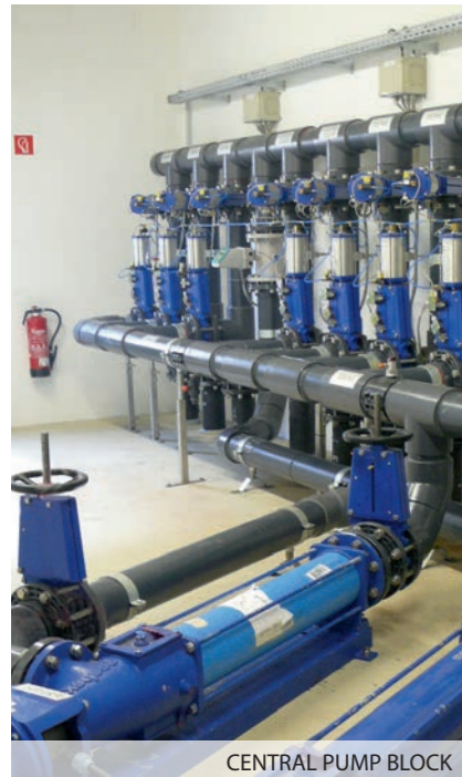
CENTRAL PUMP BLOCK
